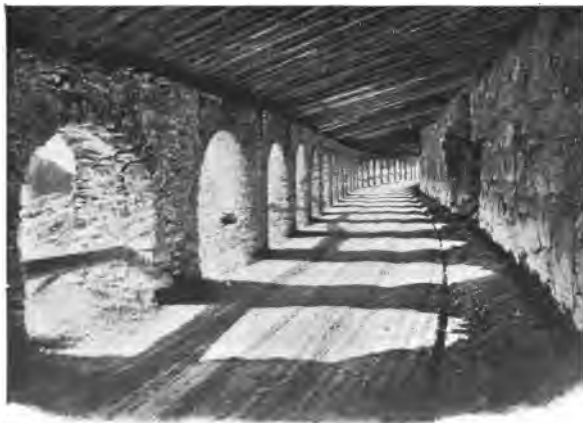
AVALANCHE GALLERIES ON THE BERNINA PASS.
